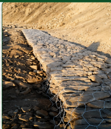
Pishin-Flood protection wall for UC Kut tehsil barshore
